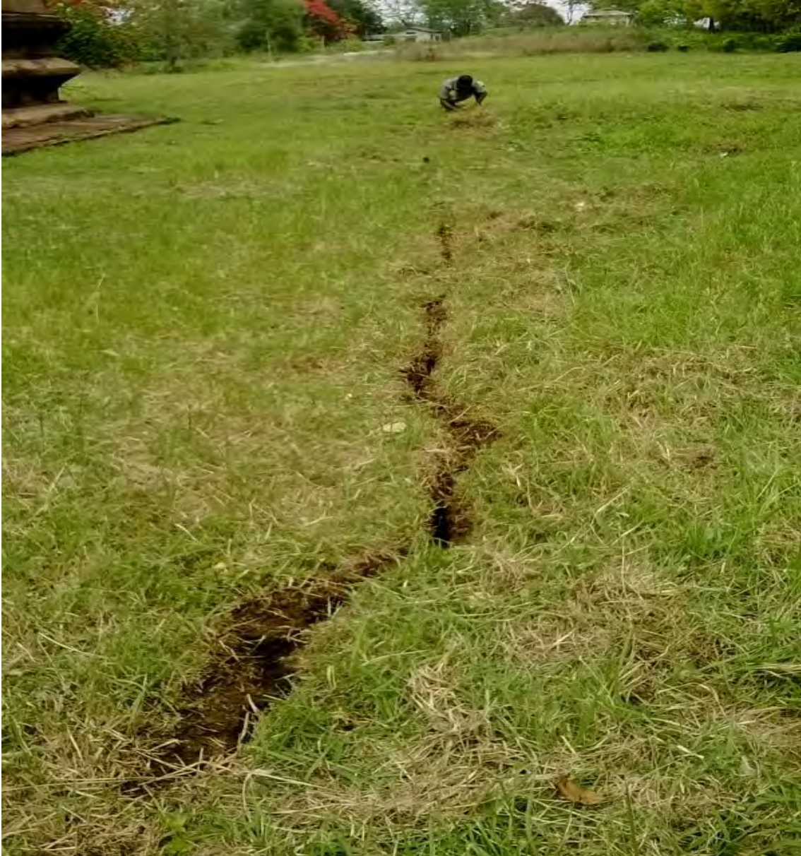
Figure 2: Earth Surface Showing the Crack
